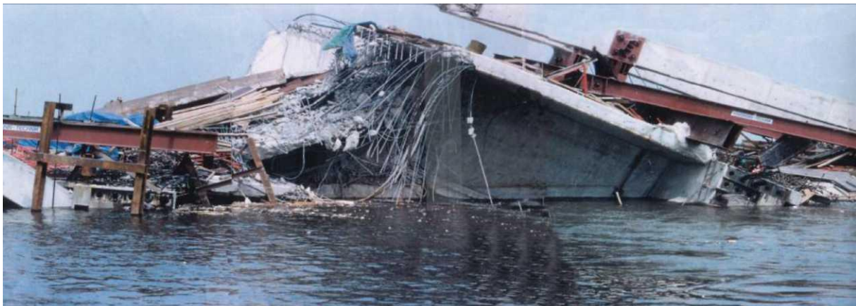
Figure 10 - Collapse of a bridge due to lacking control of the specific ground properties during pile execution (no comparison of design assumptions and locally found soil)
